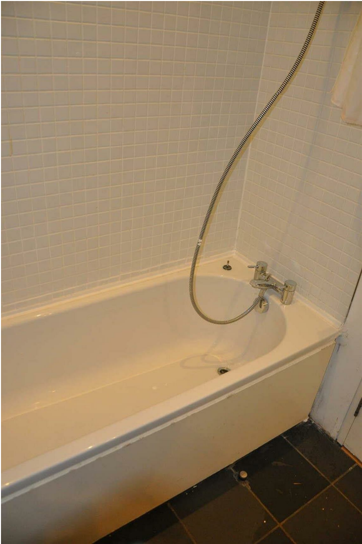
BATHROOM ANGLE TWO
