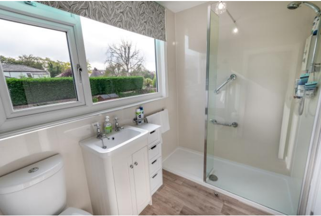
and cupboard housing wall mounted gas fired central heating boiler, hot water cylinder below and a range of shelving.
