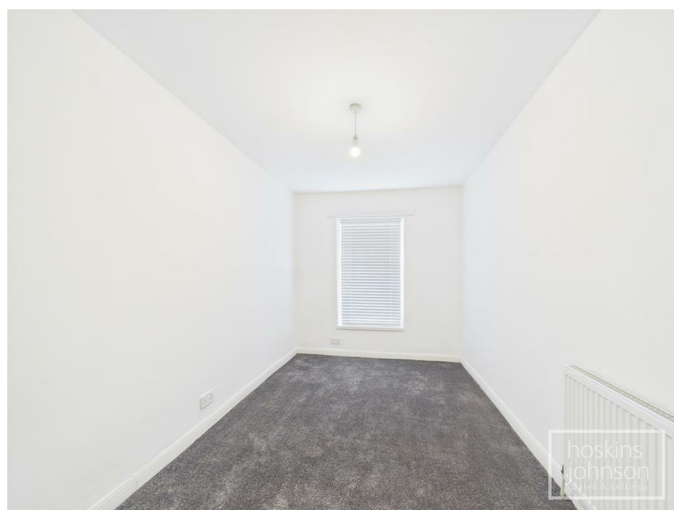
3x double plug sockets and a radiator. A window with fitted blinds.
