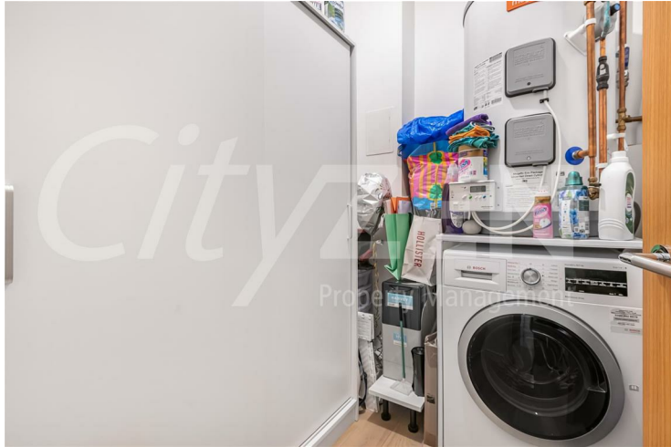
WALK IN UTILITY CUPBOARD
