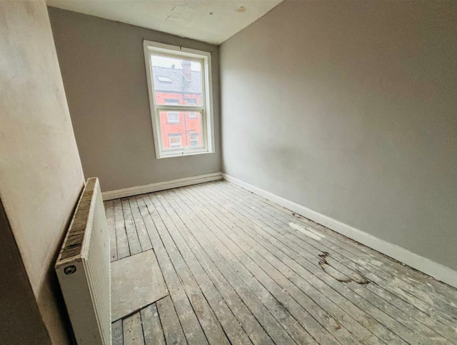
Double glazed window, central heating radiator
