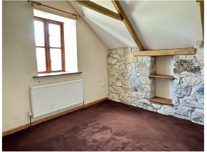
Wood frame double glazed window to front elevation with deep sill. Carpeted flooring. Radiator. Over stair recess allowing slatted storage.
