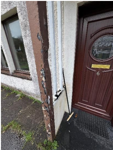
Photo 7 – Deformation of SHS post and weathering of structure
