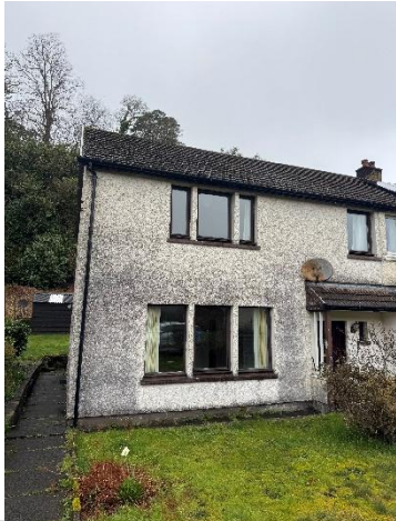
Photo 1 – Discolouration on the front elevation
