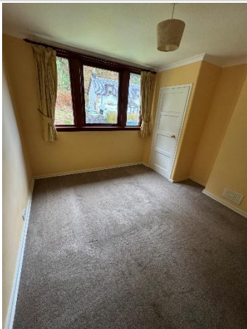
Photo 24 – Floor sloping in first floor
