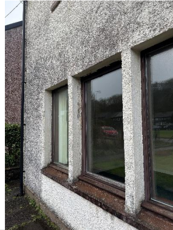
Photo 2 – Cracking noted on living room window pier
