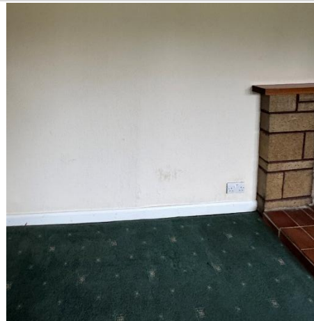
Photo 19 – Discolouration noted on internal wall in living room
