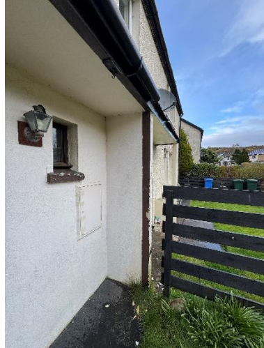
Photo 10 – Paint spalling and concrete exposed on shared wall
