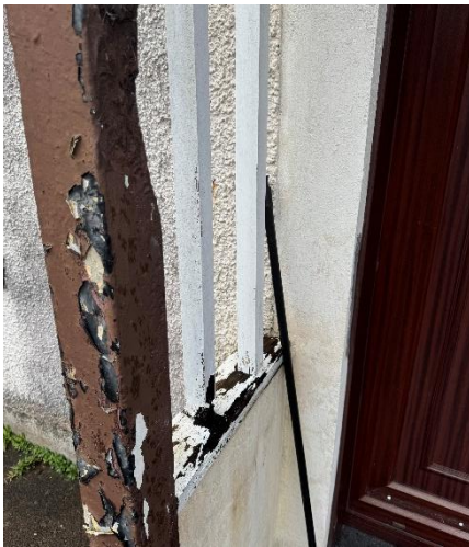
Photo 9 – Timber posts and cope rotted
