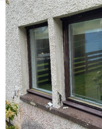
Photo 4 – Exposed reinforcement at base of kitchen window pier on the rear elevation
