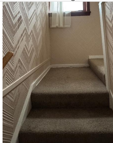
Photo 23 – Separation at skirting on landing
