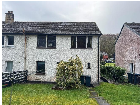
Photo 12 – Discolouration below rear windows and behind RWP
