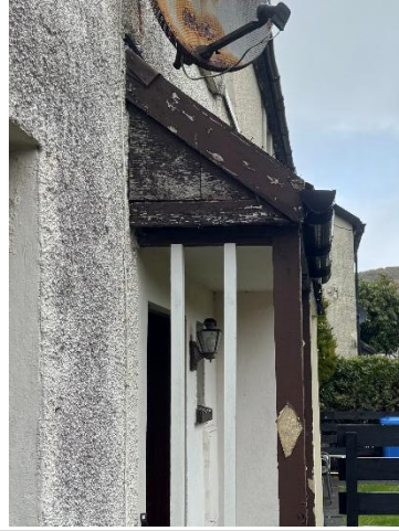
Photo 8 – Weathering of timber elements
