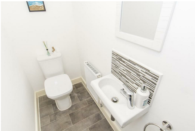
WC. Wash hand basin. Extractor fan. Radiator.
