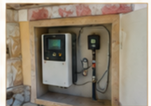
IRRIGATION CONTROL UNIT (UNDER PRINCIPAL STAIRCASE)
