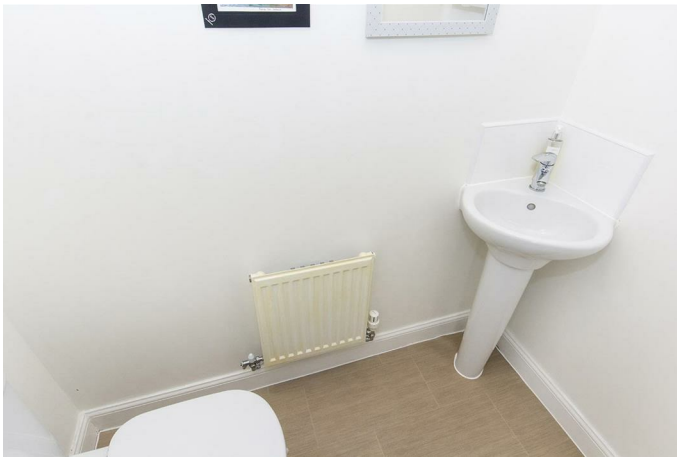
WC. Wash hand basin. Extractor fan. Radiator.
