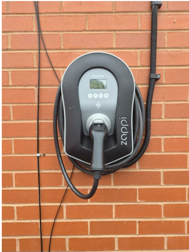
Car Recharging Point.
