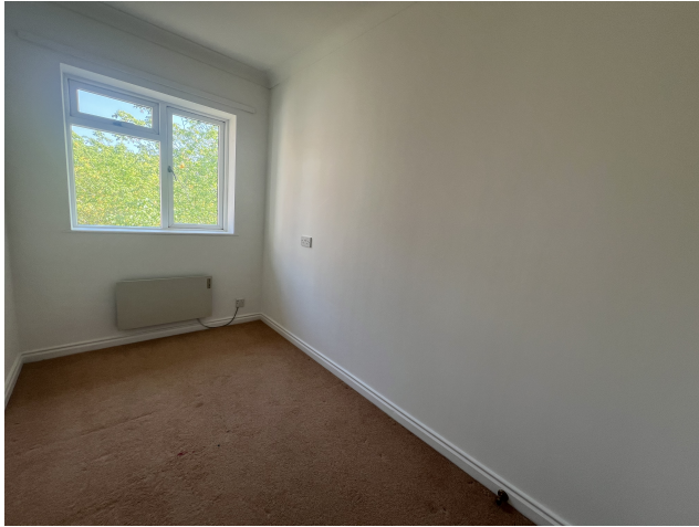
BEDROOM TWO: Double glazed windows with views over communal gardens and electric radiator.
