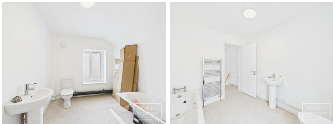
Newly fitted three piece suite in white comprising panelled bath, wc, wash hand basin, chrome heated towel rail, double glazed window to rear.
