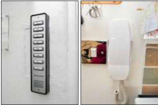
External & Internal Intercom Points
