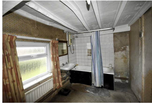
Bath, basin, low suite WC. Beamed ceiling. Airing cupboard containing the hot water cylinder and emersion heater. Radiator.
