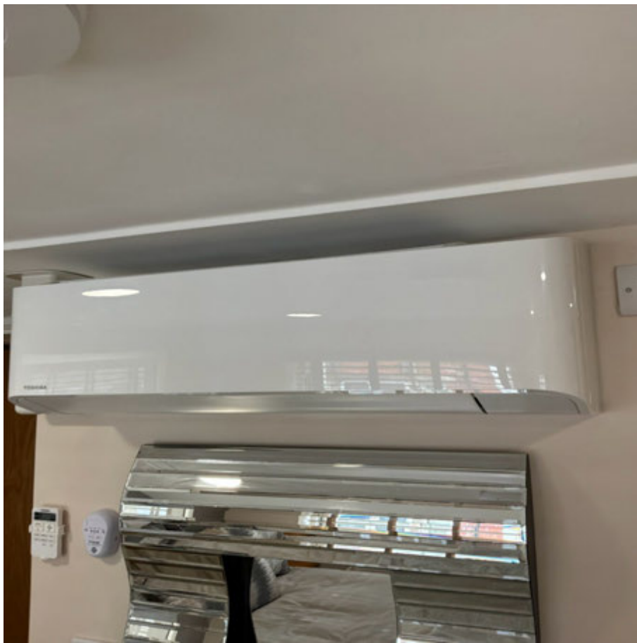
Bedroom 2 – 1 no. air conditioning unit
