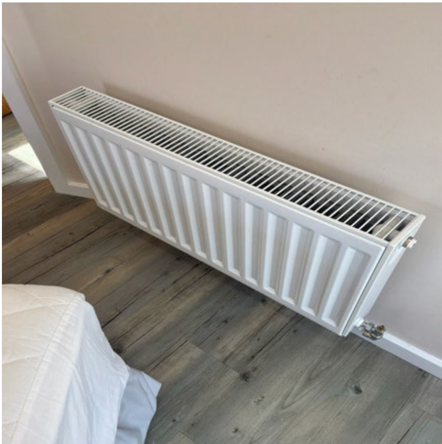
Bedroom 4 – 1 no. radiator
