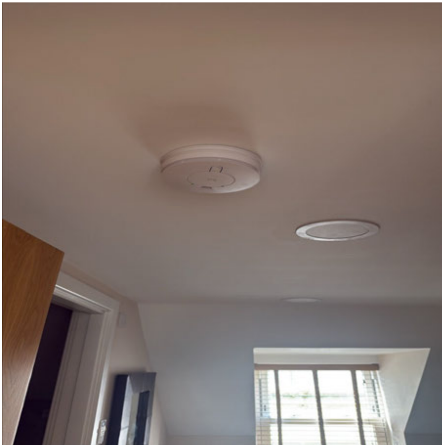
Bedroom 1 – 1 no. smoke alarm
