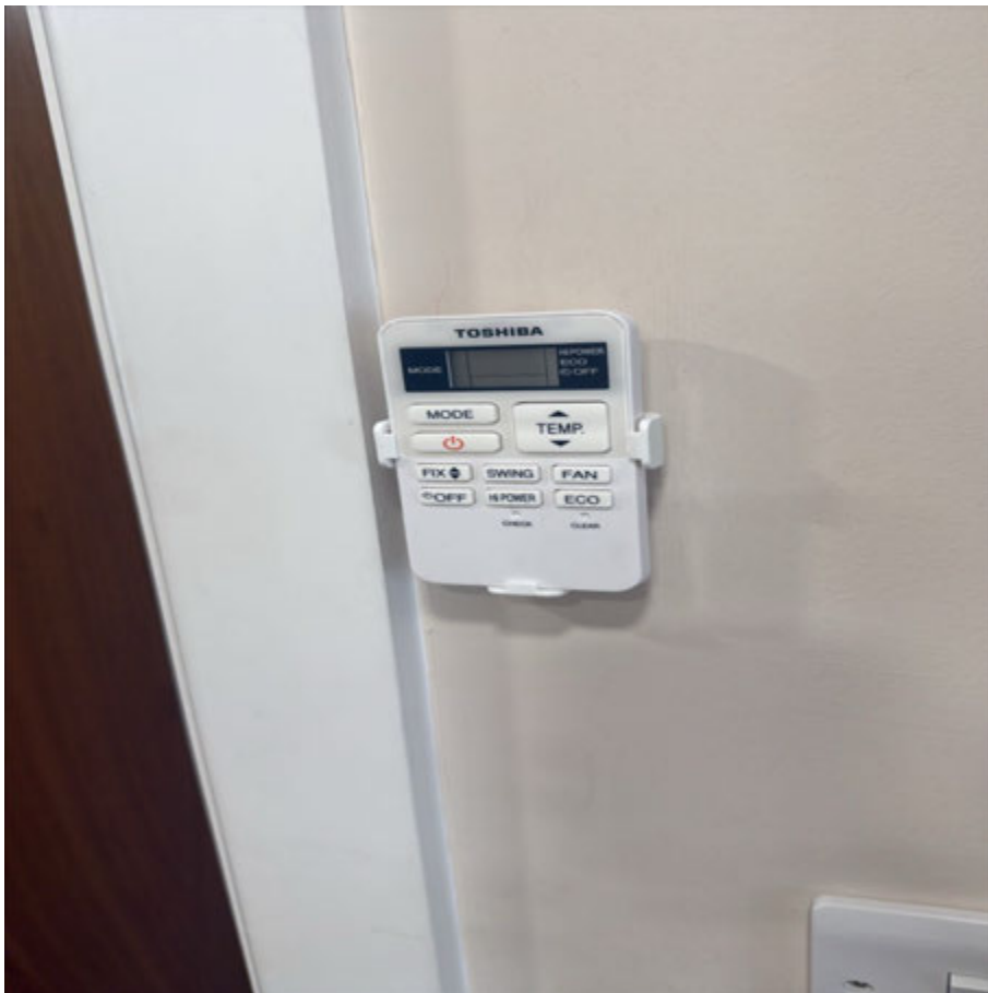
Bedroom 1 – Air Conditioning controller
