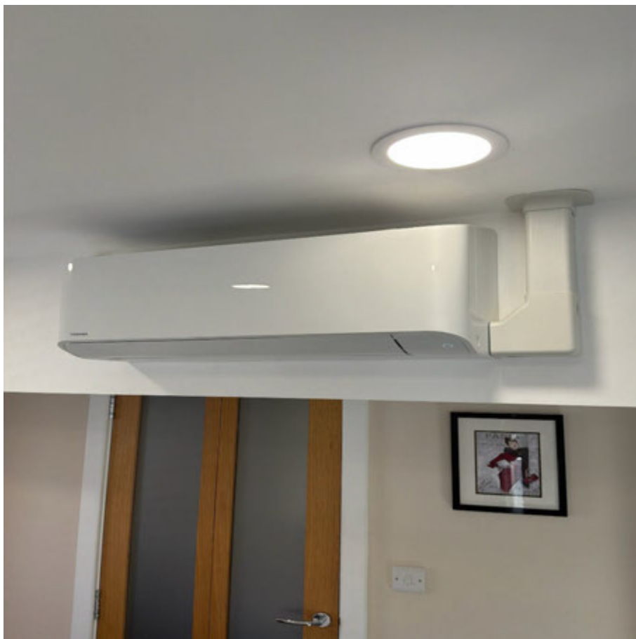
Bedroom 4 – Air conditioning unit
