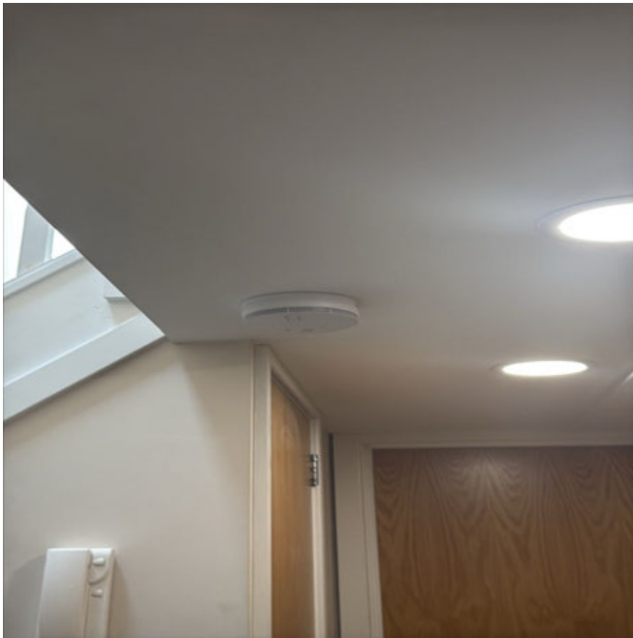
Entrance Lobby – 1 no smoke alarm
