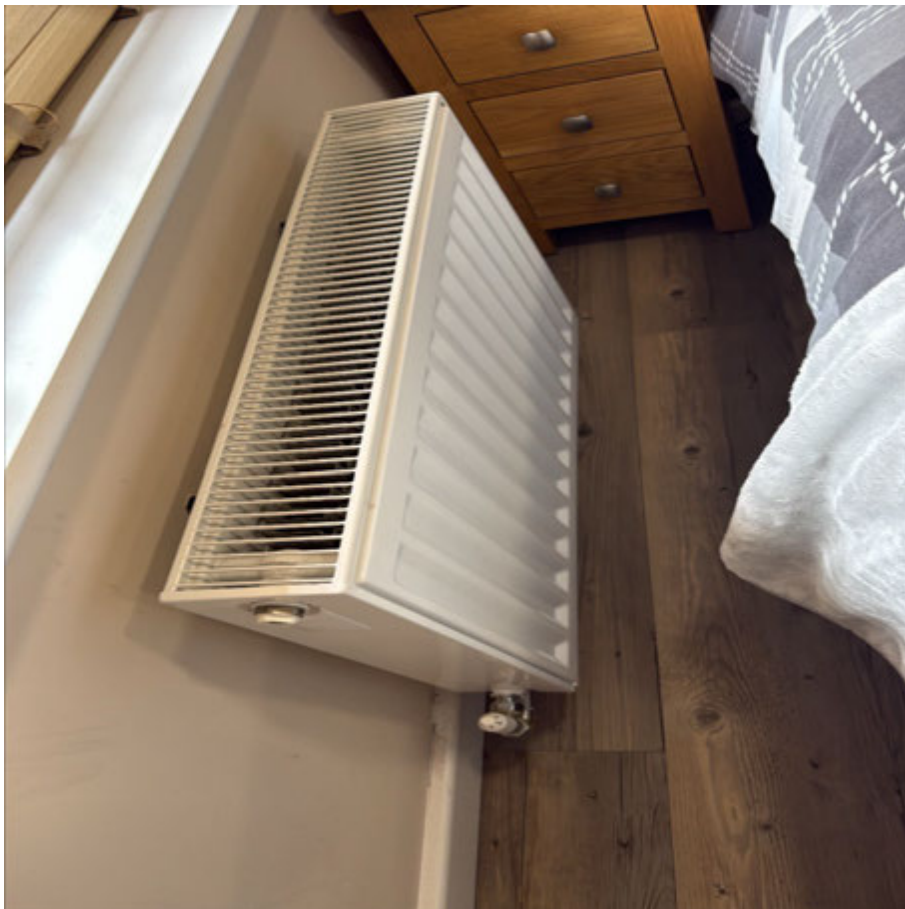
Bedroom 5 – 1 no. radiator
