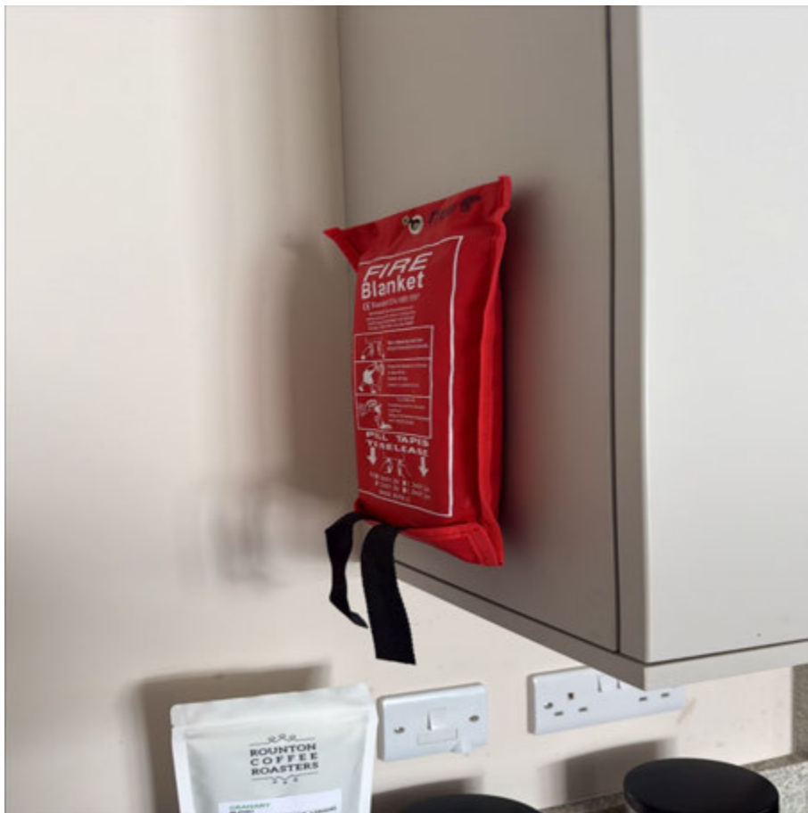
Kitchen – 1 no. fire blanket
