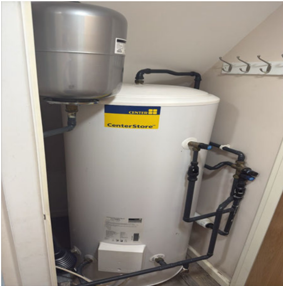
Entrance lobby – Hot water cylinder
