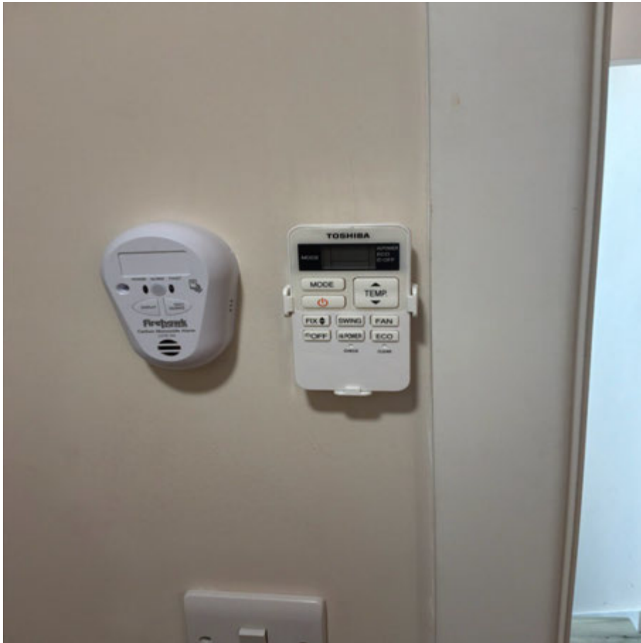
Bedroom 3 – 1 no air conditioning controller
