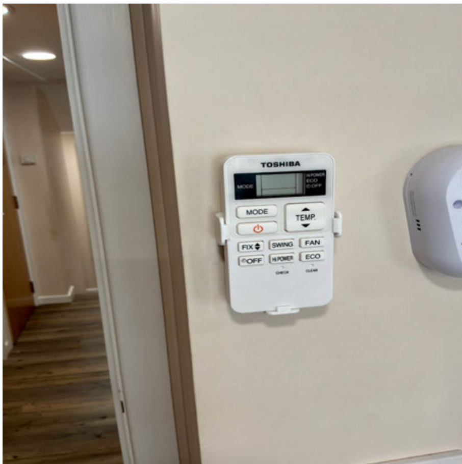
Bedroom 2 – 1 no. air conditioning controller
