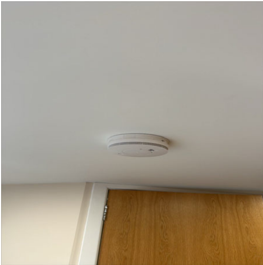
Bedroom 5 – 1 no. smoke alarm
