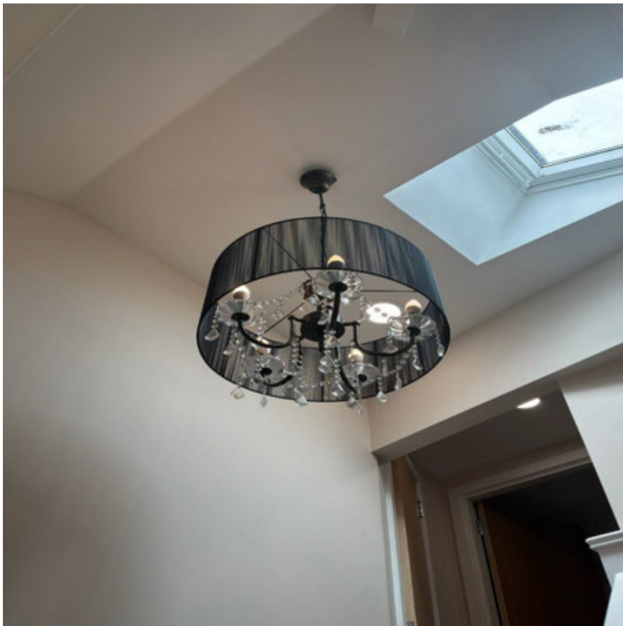
Ground floor to first floor staircase – 1 no black shade crystal light fitting
