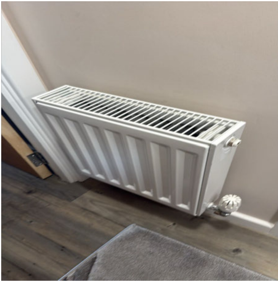
Entrance Lobby – 1 no. radiator
