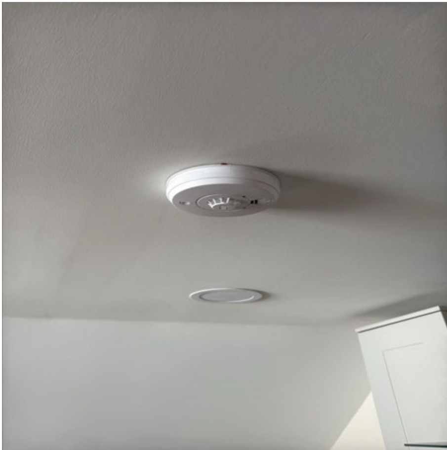
Kitchen – 1 no. smoke alarm
