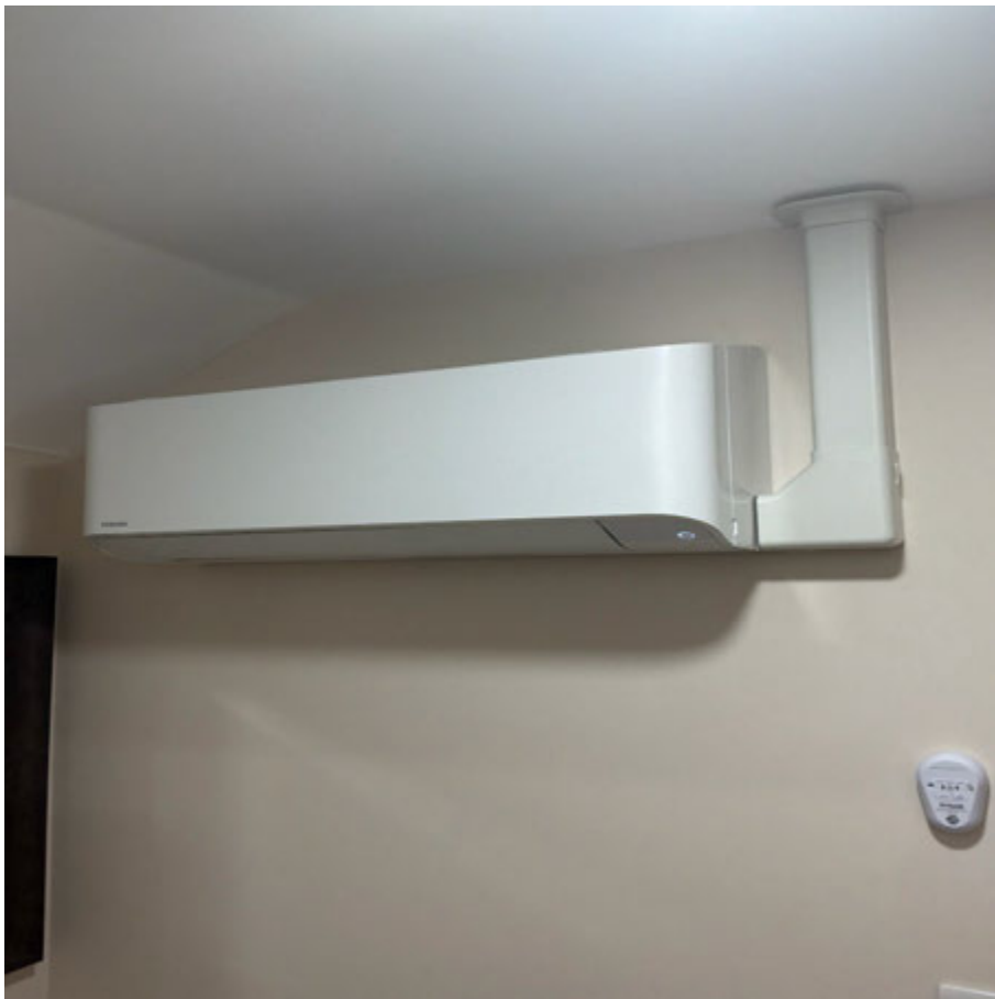
Bedroom 3 – 1 no air conditioning unit
