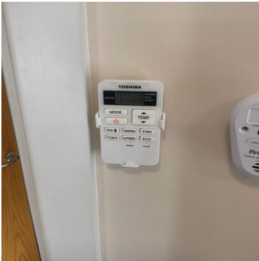
Bedroom 4 – Air conditioning remote controller
