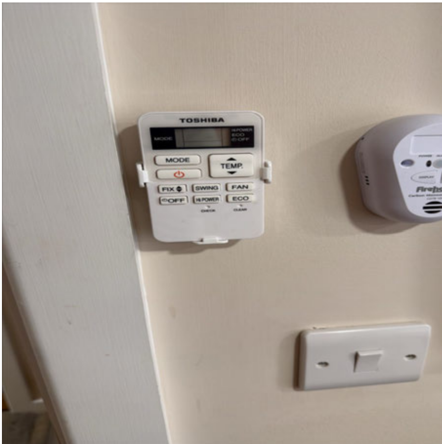
Bedroom 5 – 1 no Air conditioning controller
