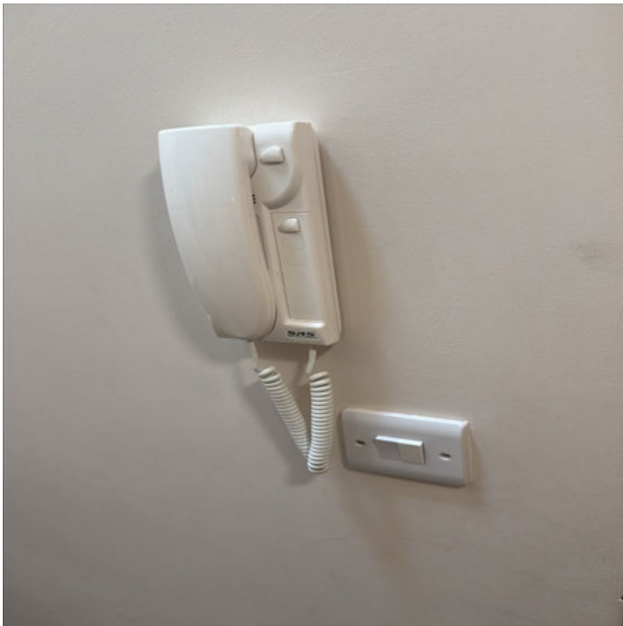
Entrance Lobby – 1 no. door entry system
