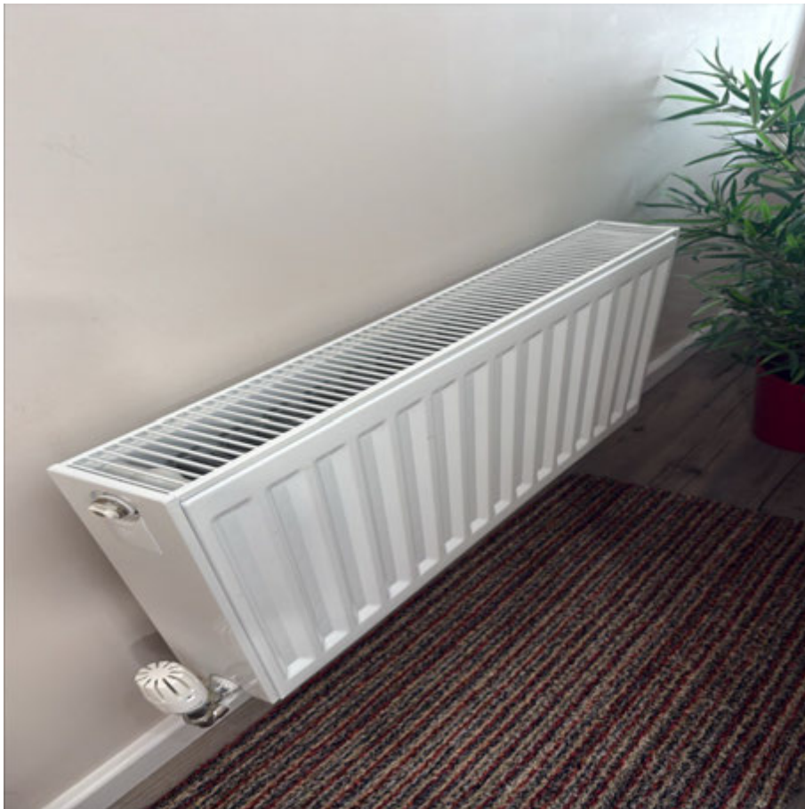
Entrance Lobby – 1 no. radiator
