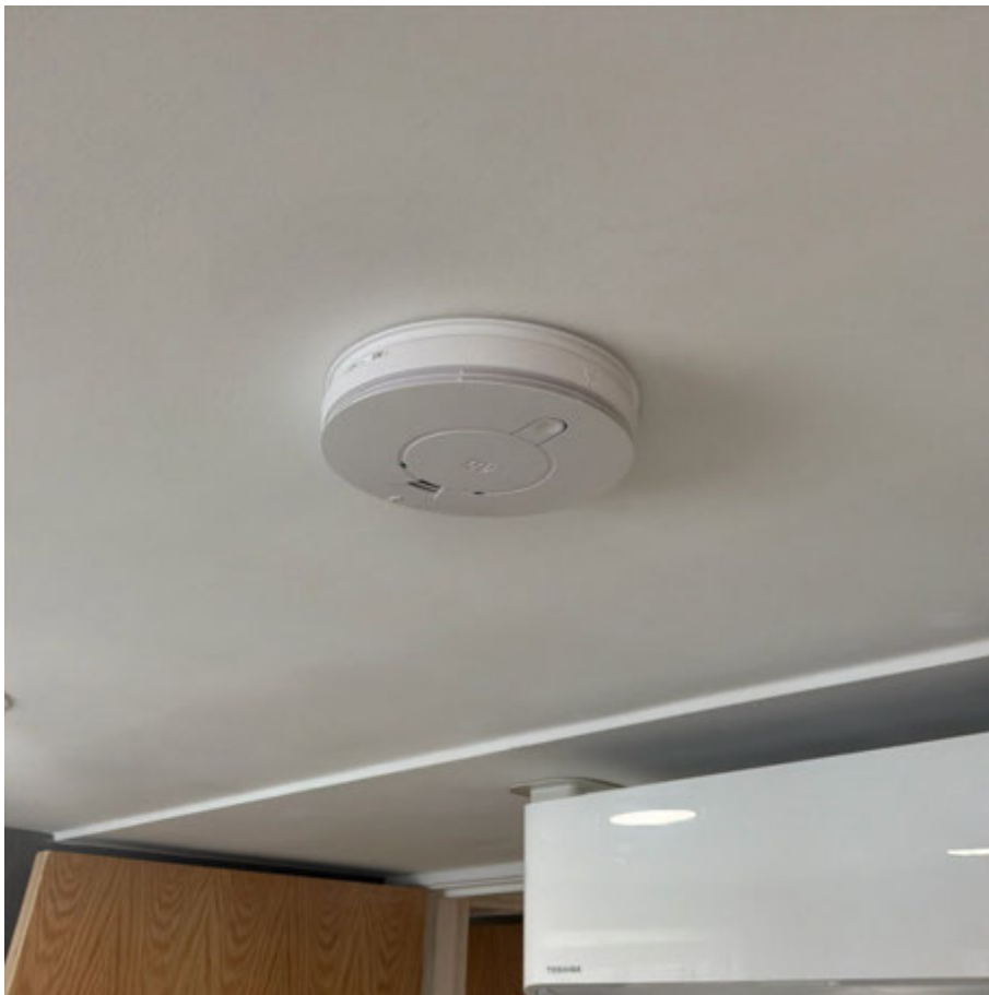
Bedroom 2 – 1 no smoke alarm in good working order
