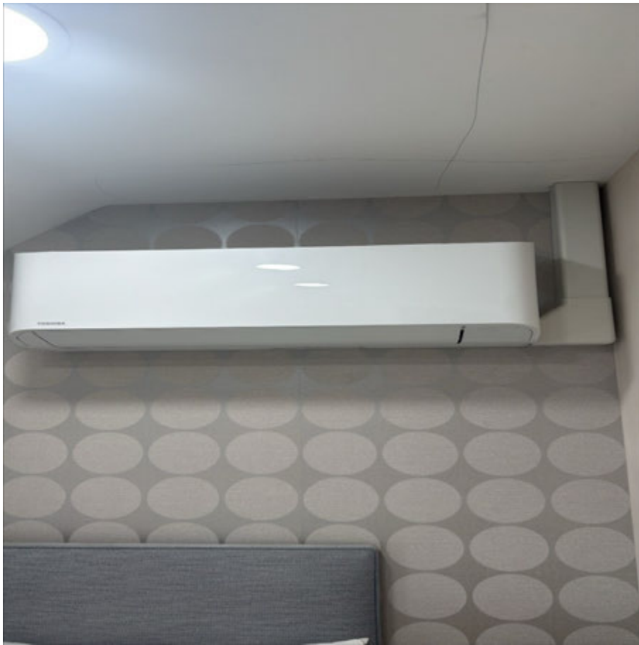
Bedroom 1 – Air Conditioning unit
