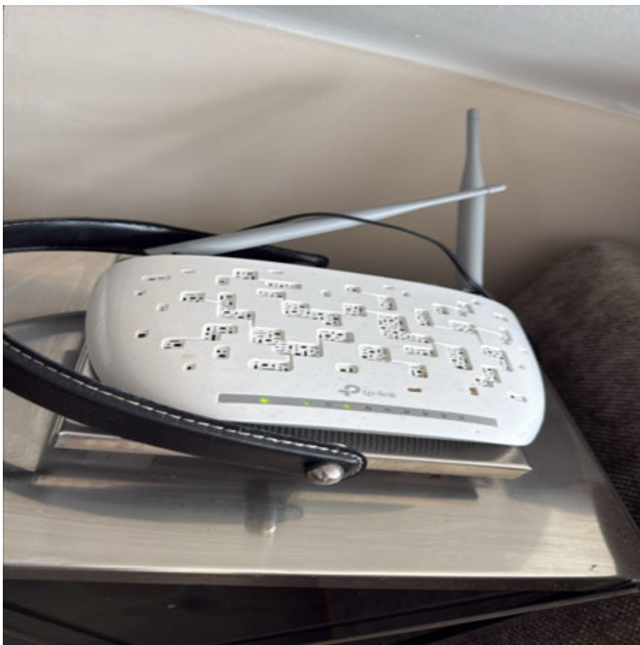
Living Room – 1 no. router
