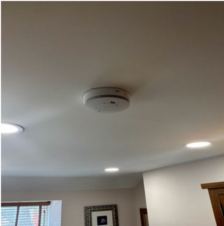
Bedroom 3 – 1 no, fire alarm in full working order
