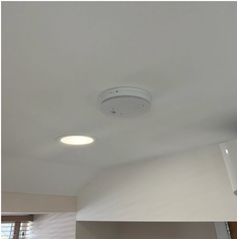
Bedroom 4 – Fire alarm in fully working order
