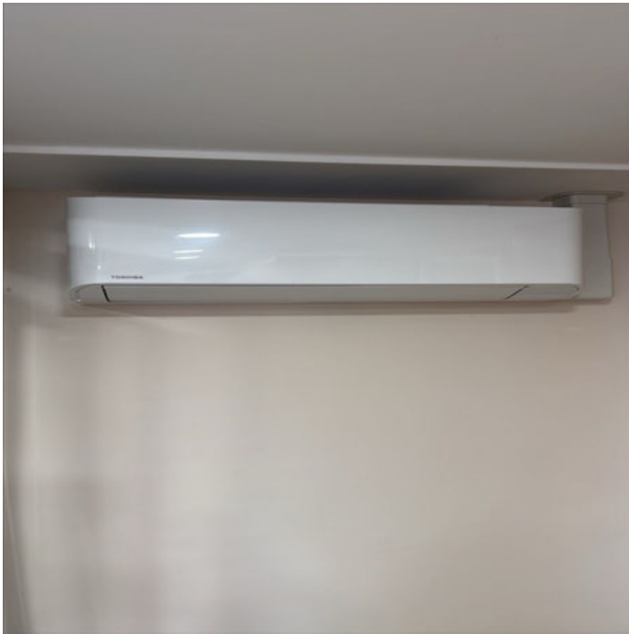
Bedroom 5 – 1 no. air conditioning unit
