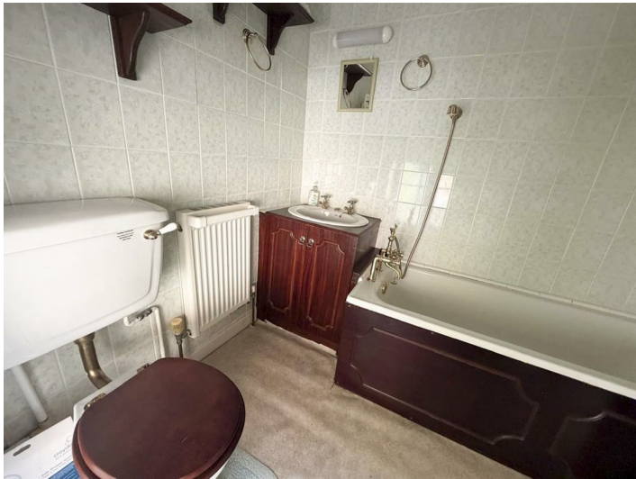
Wash handbasin set in bathroom furniture, WC, bath with mixer tap and shower over. Heat/Light unit, radiator, obscured window to rear.
