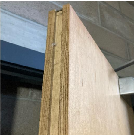
Figure 9—3 Seals missing from fire doors
