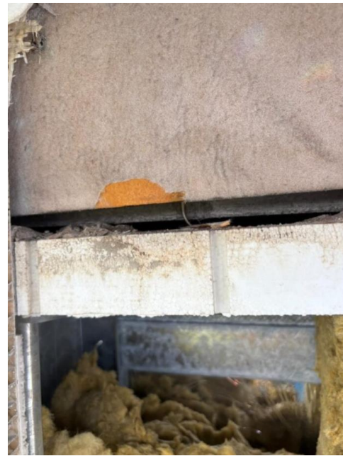
Figure 5—4 Evidence photo 3. Phenolic insulation present at slab edge.
