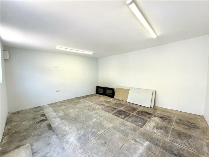
double glazed window - wall mounted consumer unit - partially paved floor covering.
