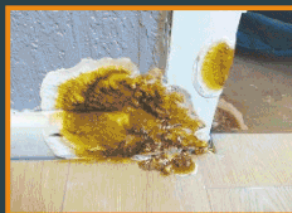
Wet & Dry Rot Control
