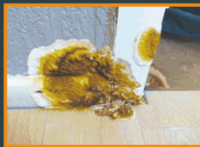
Wet & Dry Rot Control
