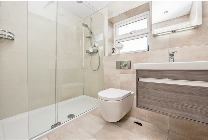
Used as an en-suite shower room for bedroom one / a family shower room: Double glazed window, a modern white suite comprising of a walk-in shower area with a glazed side screen and a plumbed shower, wash basin set into a vanity unit, low flush WC with a concealed cistern, modern tiling, extractor fan, ladder style central heating radiator / towel warmer
