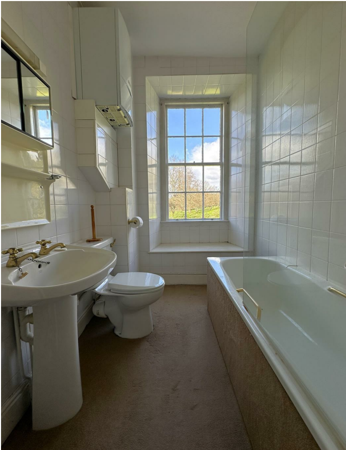
Sash window, window seat, bath, wash hand basin, toilet and wall mounted gas fired boiler.
