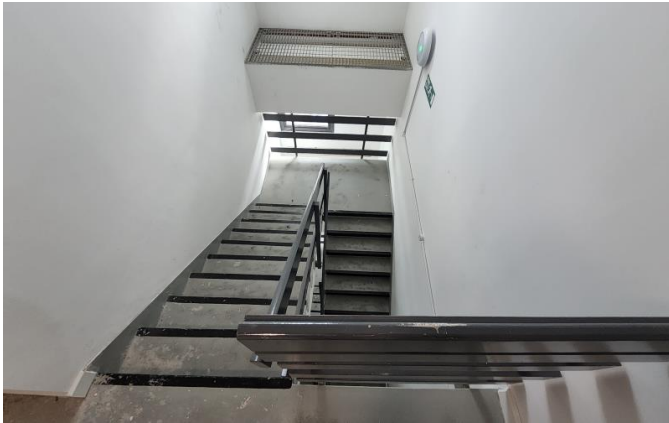
Handrails are fitted to the internal stairs.
