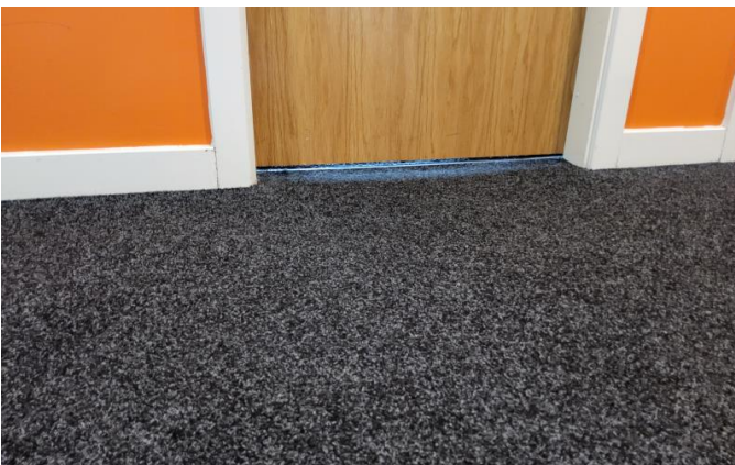
Room 6-01's front entrance door with gaps that exceed the recommended tolerances.
