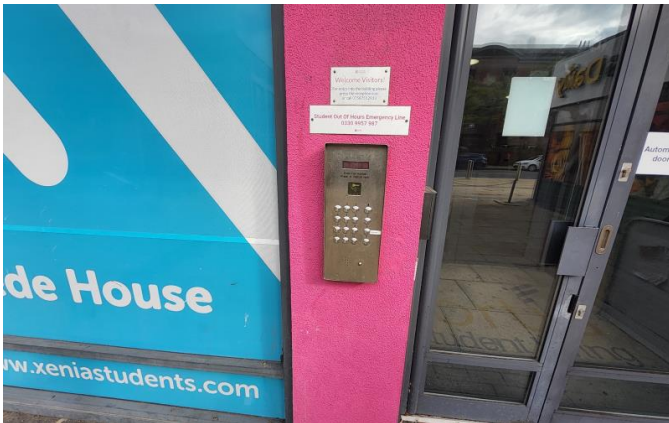
Occupier-operated intercom system.
