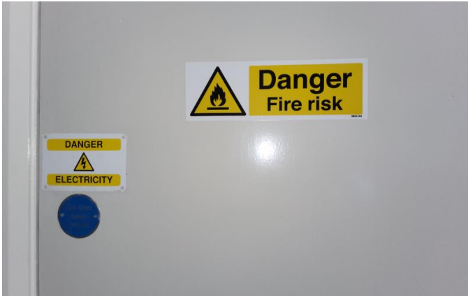
Electrical hazard signs.
