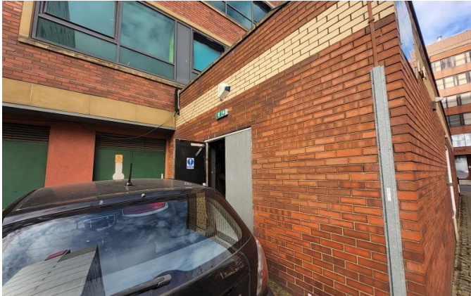
Lightning protection system.
