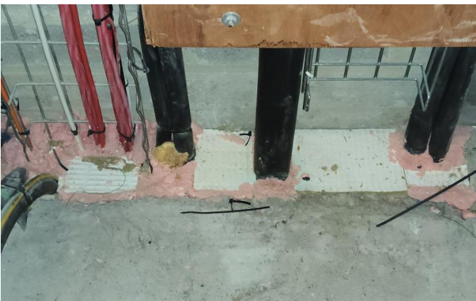
Expanding foam used to fire-stop gaps in the riser cupboards.
