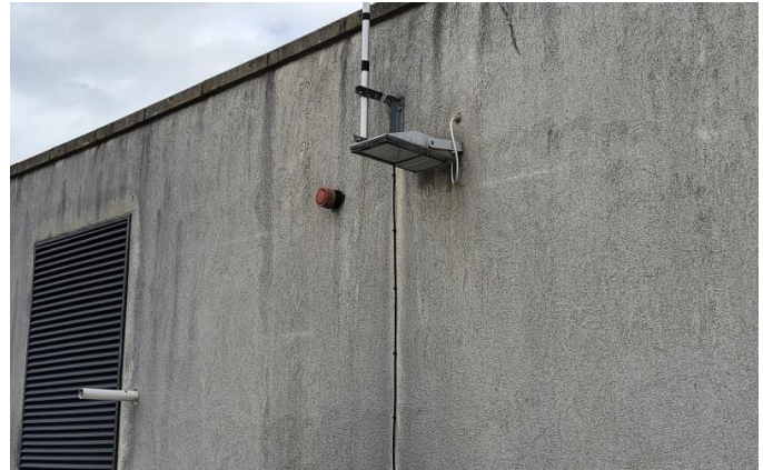
Example of a sounder unit on the flat roof.
