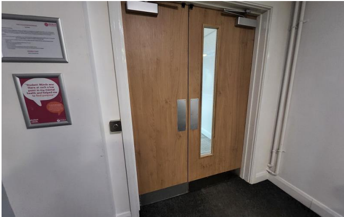
Ground floor lobby doors with no signs visible.
