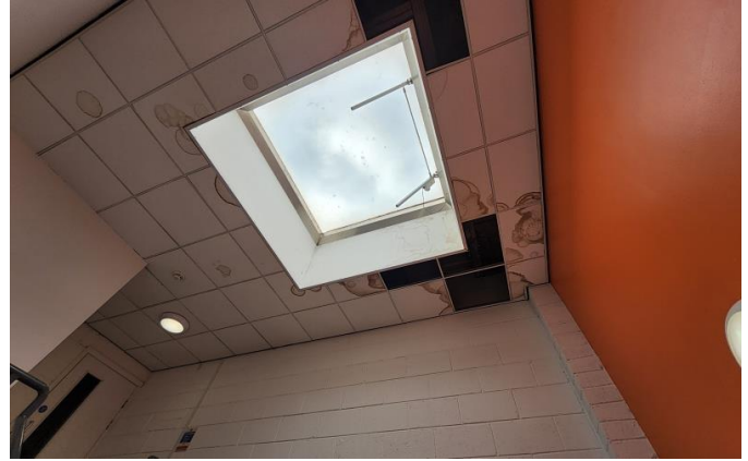
Damaged and missing ceiling tiles in the protected stair.
