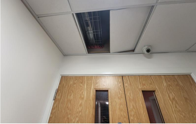
Expanding foam used to fire-stop gaps between compartments.
