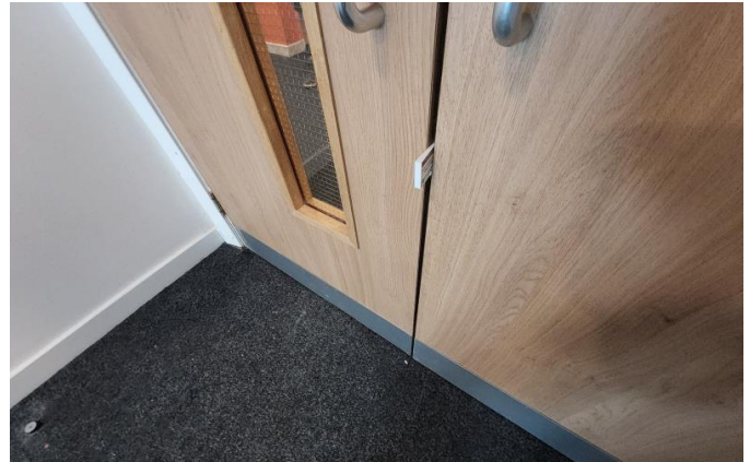
Example of a lobby door with gaps that exceed the recommended tolerances. .
