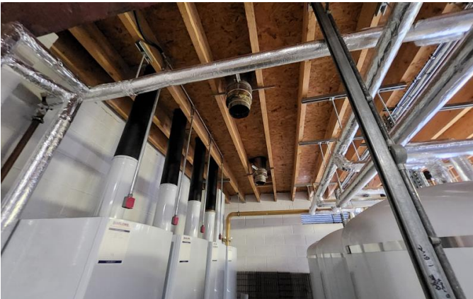
Incomplete compartmentation with exposed beams in the boiler room.
