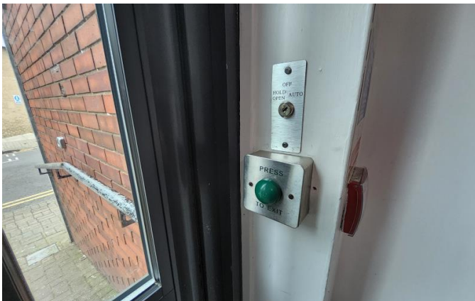
Rear fire exit door's electronic release switch.
