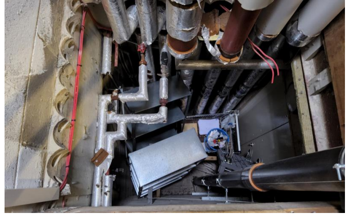
Example of combustible waste in the riser cupboards.
