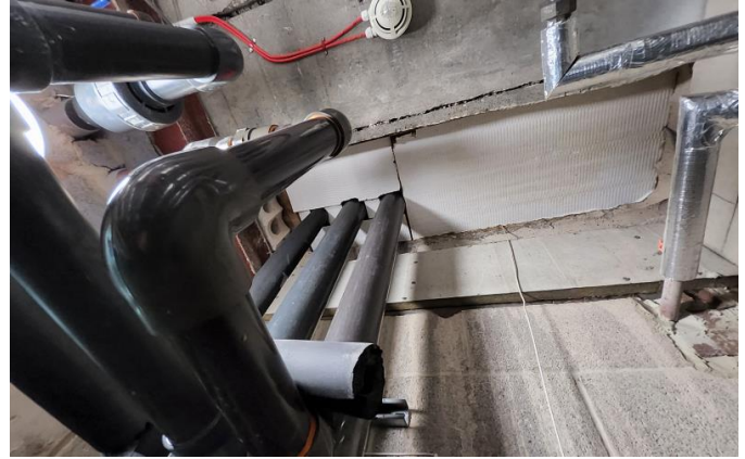
Incomplete compartmentation in the riser cupboards.
