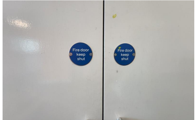
Incorrect signs on the riser cupboard doors.
