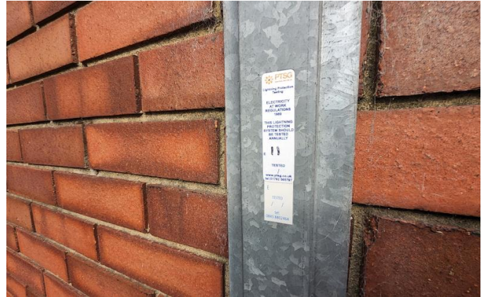
Lightning protection system.
