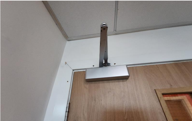
Example of a fire-rated lobby door's positive self-closing device.
