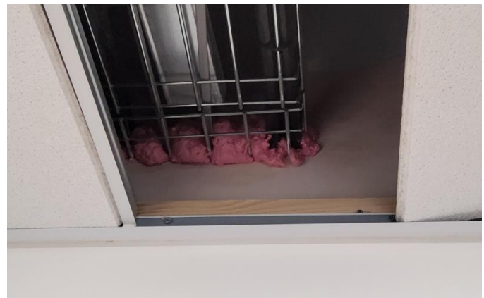
Expanding foam used to fire-stop gaps between compartments.
