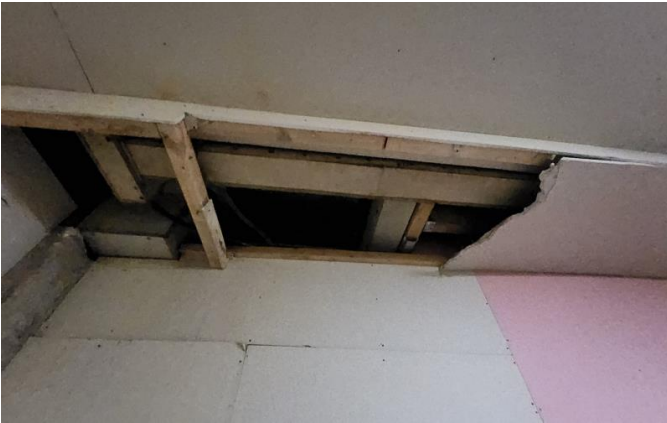
Damaged ceiling in the bike store.
