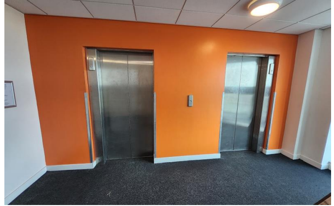
Example of a lift in the common areas missing a "Do not use life is event of fire' sign.
