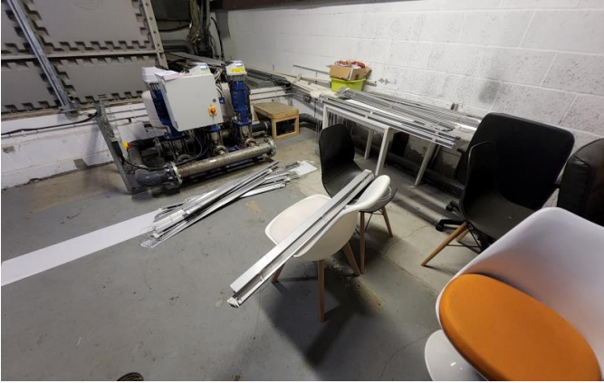
Combustible waste in the water tank room.
