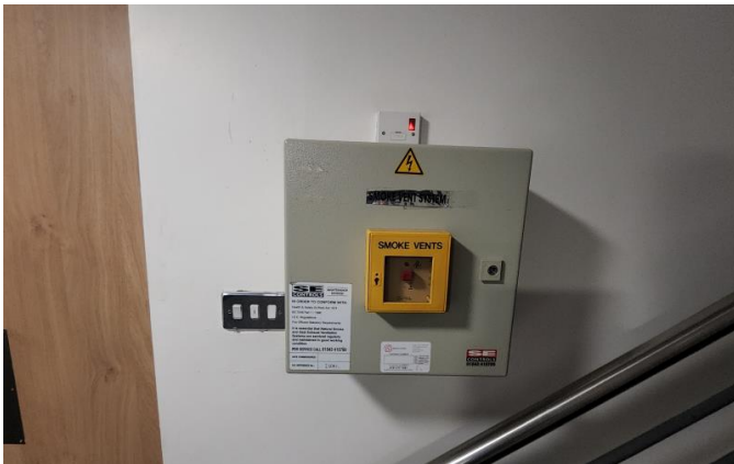
Smoke Vent Swich Control Panel.
