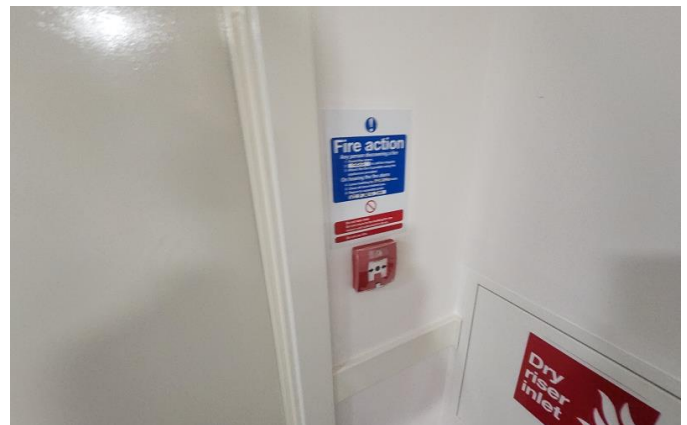
Example of a manual call point next to the final exits.
