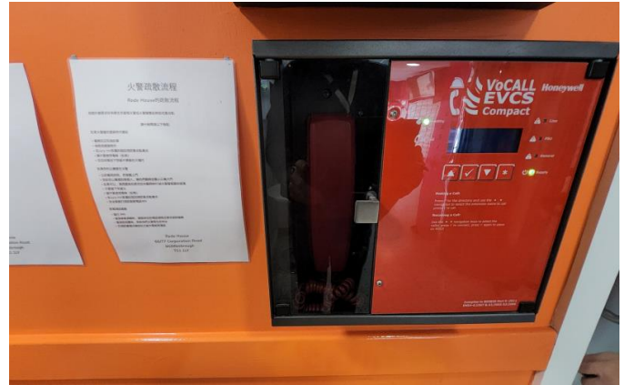
Refuge fire point system.
