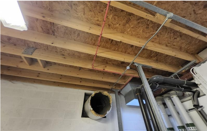
Incomplete compartmentation with exposed beams in the water tank room.
