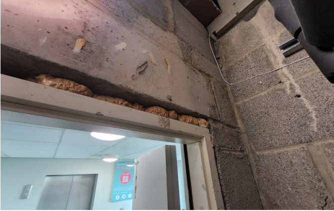
Incomplete compartmentation around the riser cupboard doors.
