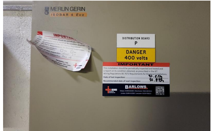
Electrical inspection label dated 21/08/2024.
