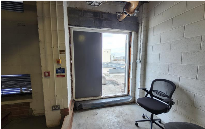
Roof access door was unlocked.
