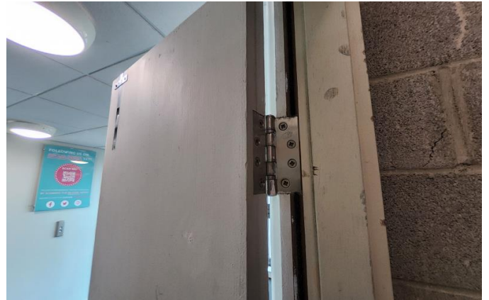
Example of a riser cupboard door's fire-rated hinges and combined intumescent strips with cold smoke seals.
