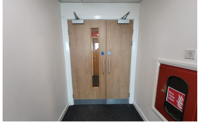
Example of a fire-rated lobby door.
