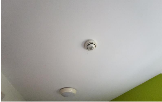
Example of a smoke alarm in flat 6-01.
