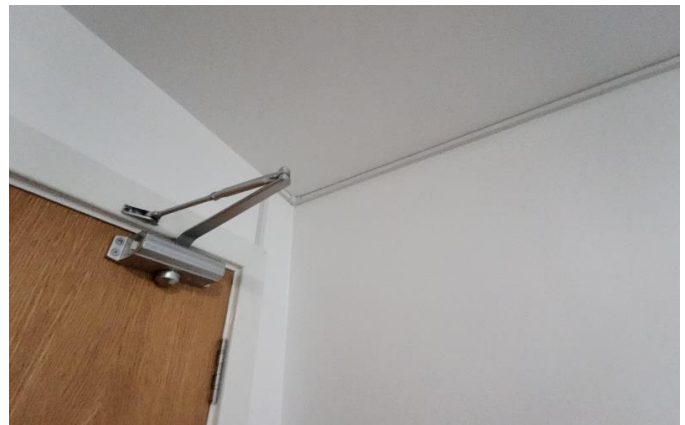
Example of plastic electrical conduit above flat 02-39's front entrance door.
