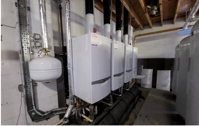
Gas combi-boilers in the plant room.
