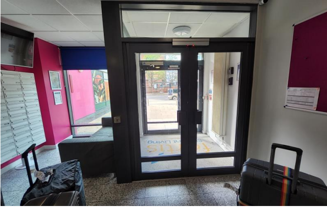
Fire exit signs are missing from above the final exit doors.
