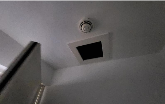
Missing access hatch in the 5th floor storeroom.
