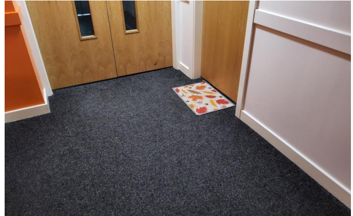
Example of doormats on the escape routes in the common corridors.
