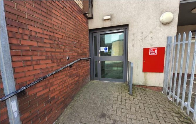
Fire exits are missing the 'Fire exit keep clear' sign on the doors.
