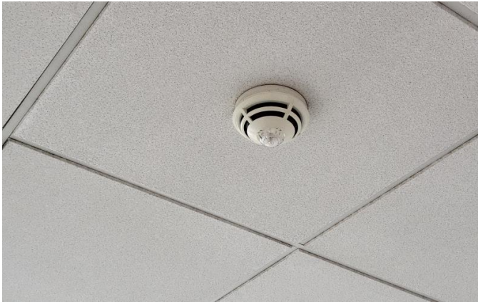
Example of a smoke alarm in the common areas of the building.
