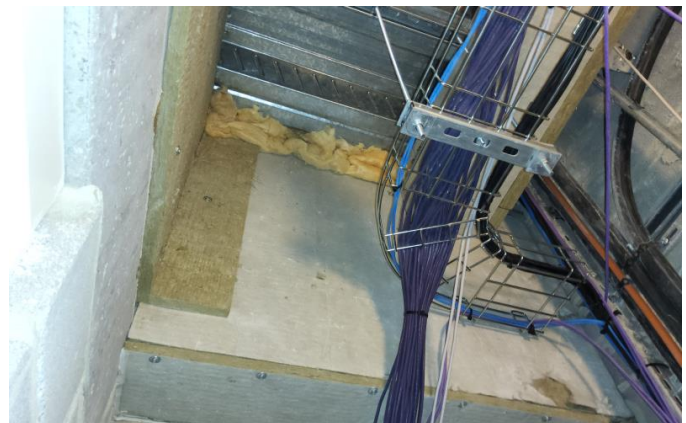
Incomplete compartmentation in the laundry room riser cupboard.
