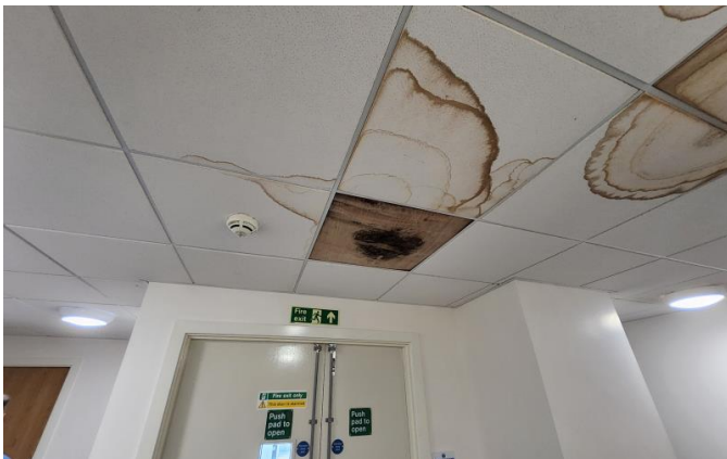
Damaged ceiling tiles in the common corridors.
