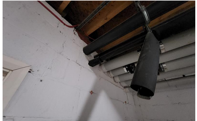
Evidence of fire-stopping in the plant room.
