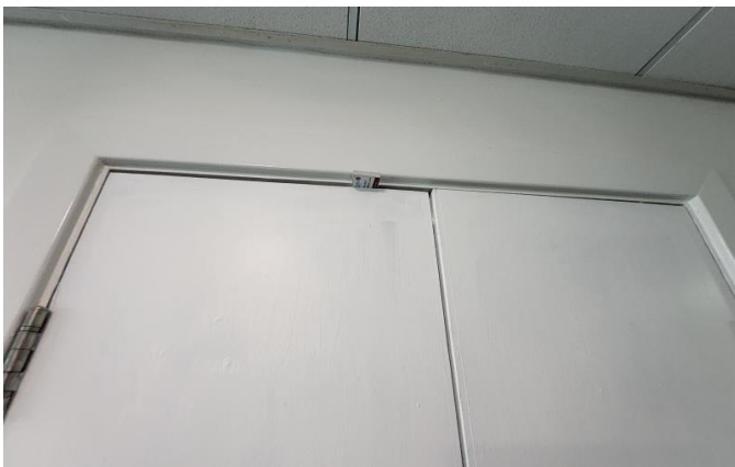
Riser cupboard door with gaps that exceed the recommended tolerances.
