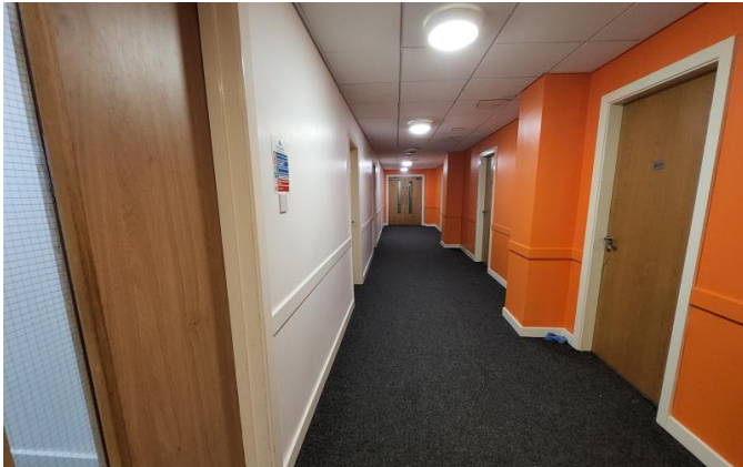
Internal emergency lighting.
