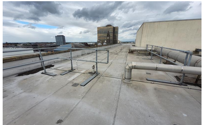
'Mansafe' roof system installed.
