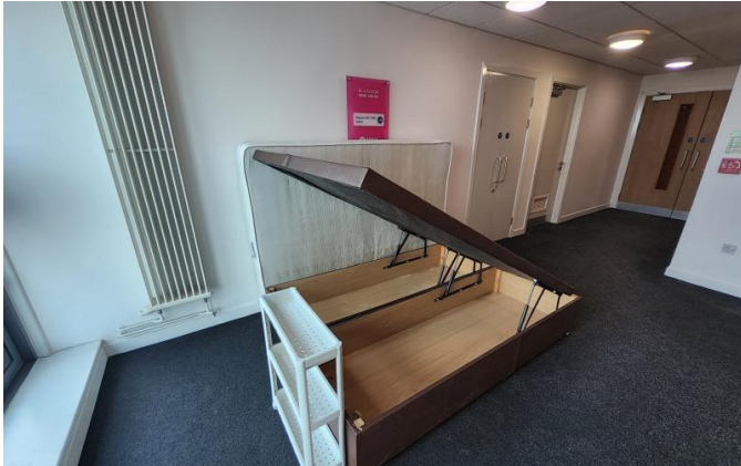
Furniture on the 6th floor escape route.
