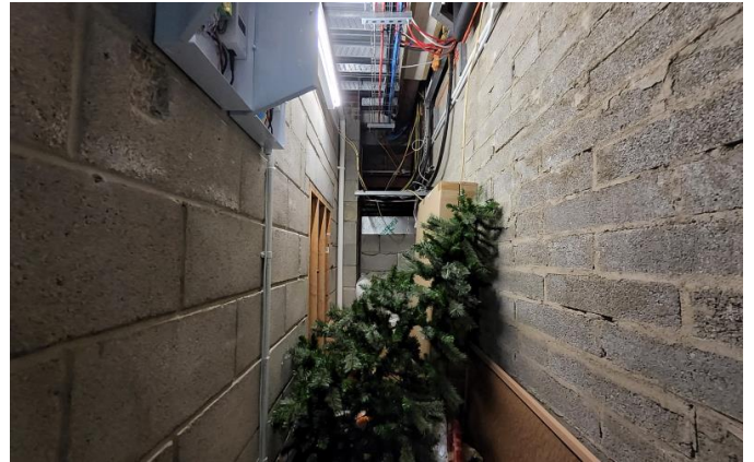
Combustible waste in the ground floor storeroom next to the cloakrooms.
