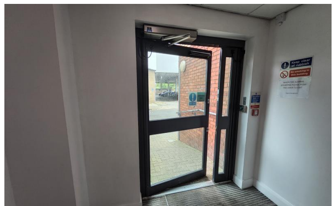
Fire exit signs are missing from above the final exit doors.
