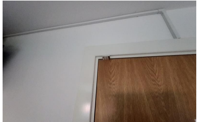
Room 6-01's front entrance door with gaps that exceed the recommended tolerances.
