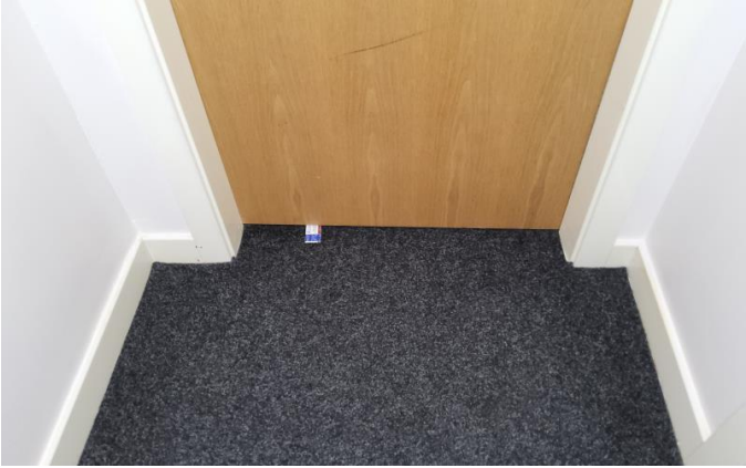
Room 2-39's front entrance door with gaps that exceed the recommended tolerances.
