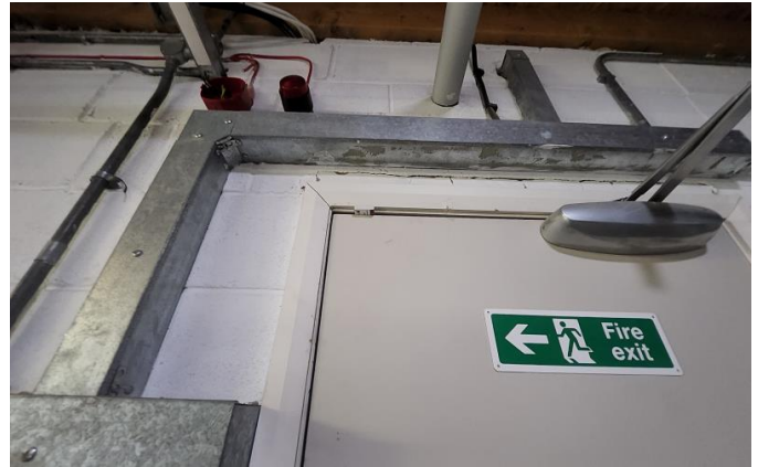
Example of a plant room door with gaps that exceed the recommended tolerances.
