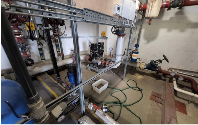
Water pumping equipment.
