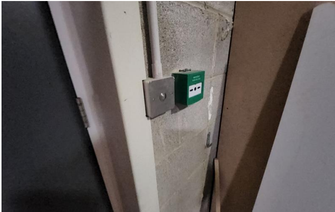
Electronic exit with emergency break glass point in the cycle store.
