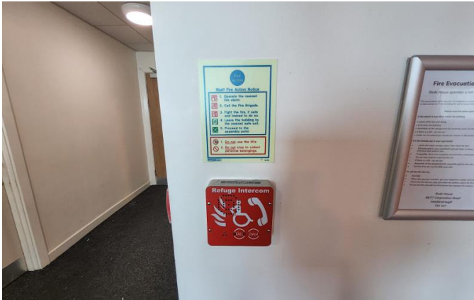
Refuge fire point.
