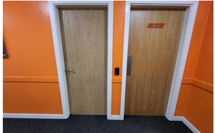
Kitchen and cloakroom doors with no signs visible.
