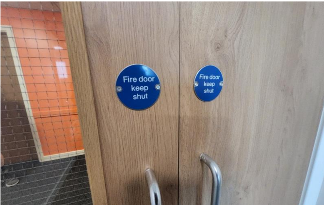
'Fire door keep shut' signs on the riser lobby doors.
