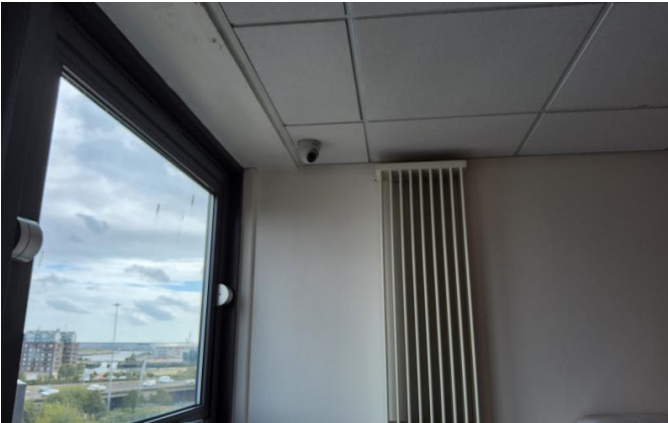
Example of a radiator in the common corridors.
