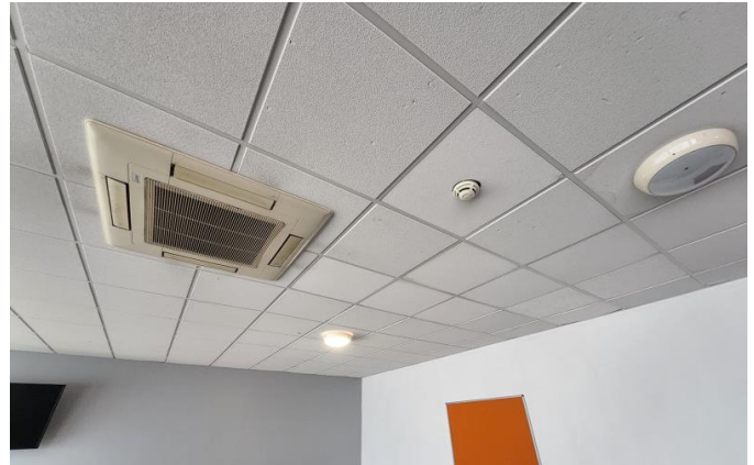
Example of an air-conditioning system in the communal areas.
