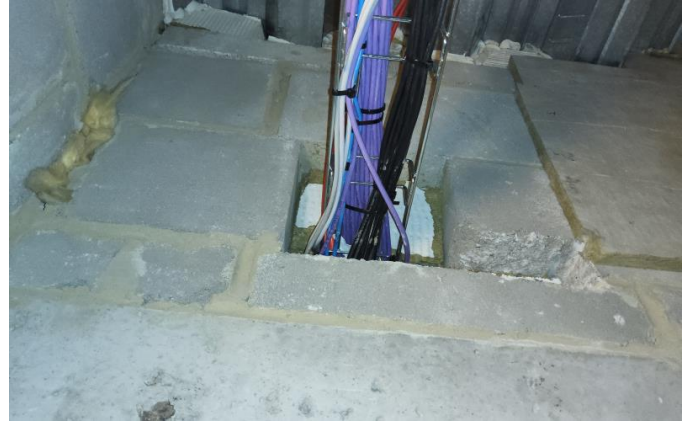
Incomplete compartmentation in the riser cupboards.
