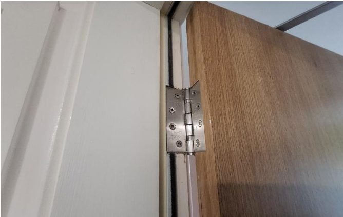
Room 6-01's front entrance door's fire-rated hinges and combined intumescent strips with cold smoke seals.
