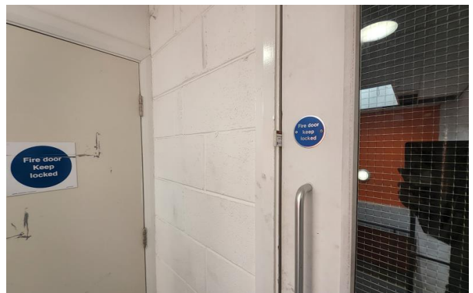
'Fire door keep locked' signs on the plant room doors.
