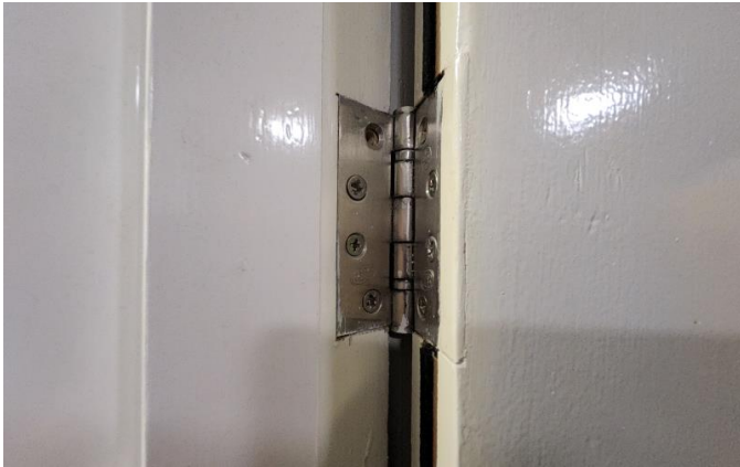
Example of a riser cupboard door with screws missing from the hinges.
