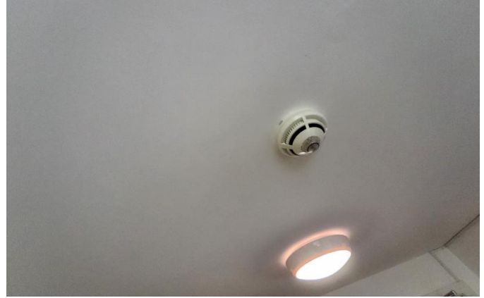
Example of a smoke alarm in flat 2-39.
