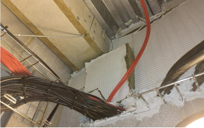
Incorrect levels of fire-stopping in the riser cupboards.
