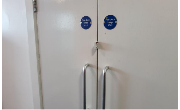
Riser cupboard door with gaps that exceed the recommended tolerances.
