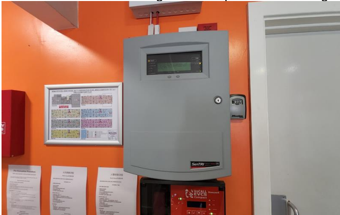
Fire alarm panel with a zone plan in the entrance lobby.
