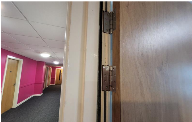
Example of a lobby door with seals missing.
