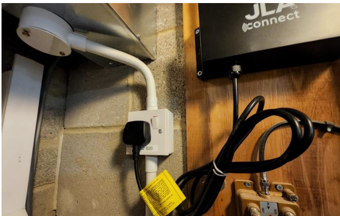
Example of un-tested AV equipment in the riser cupboards.
