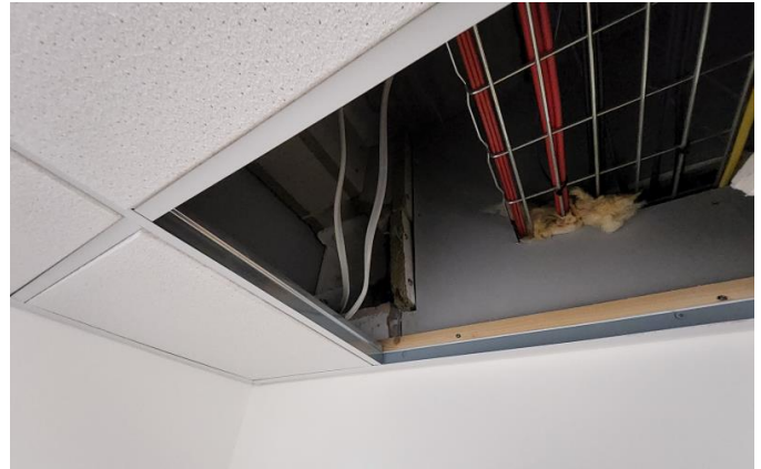
Incomplete compartmentation above the cross-corridor door.
