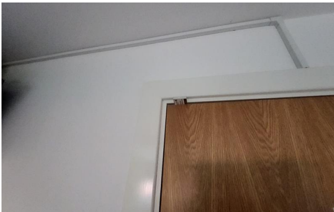
Example of plastic electrical conduit above flat 06-01's front entrance door.
