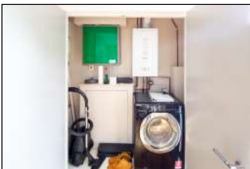
Utility, Plant & Communications Cupboard
