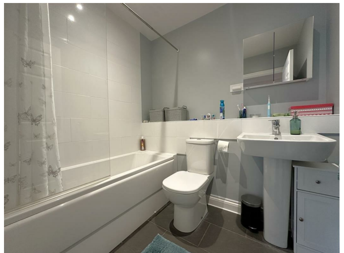
Extractor fan, towel radiator, toilet, wash hand basin and bath with shower screen and shower over.
