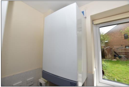
Central Heating Boiler
