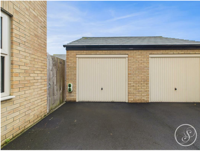
Power and lights.
