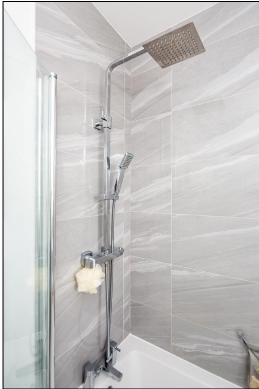
Bathroom – rain head shower over the bath
