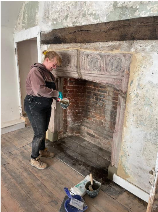
Conservator Emma Teale, of the Skillington Workshop, carrying out mortar repairs to the Elizabethan fireplace.
