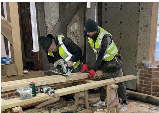
Ron and Lee of Dock and Cottee Carpentry carrying out timber-frame repairs in the hall
