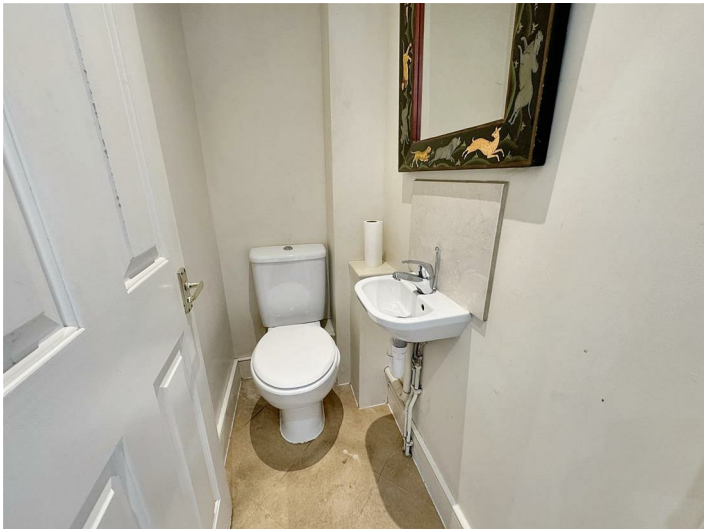
low flush w/c - wall mounted wash basin.
