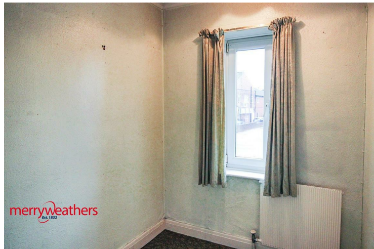
Front UPVC Window and central heating radiator.
