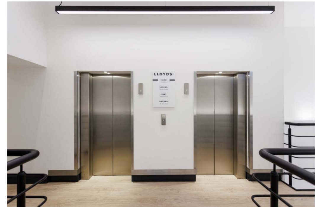
2 X 8 PASSENGER LIFTS
