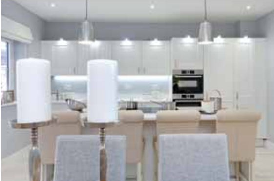
Low energy pendant lights and LED downlights
