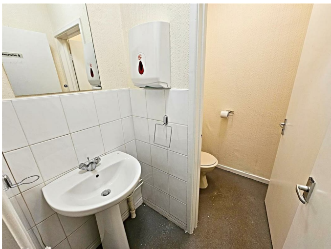
WC, wash hand basin, part tiled walls, double glazed window to side.
