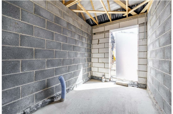
Door to side aspect. The layout will comprises of base units with plumbing for washing machine and space for tumble dryer.
