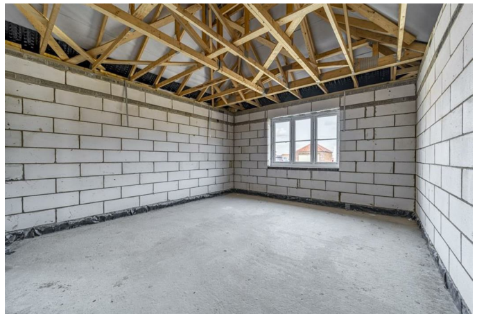
Upvc window to front aspect.
