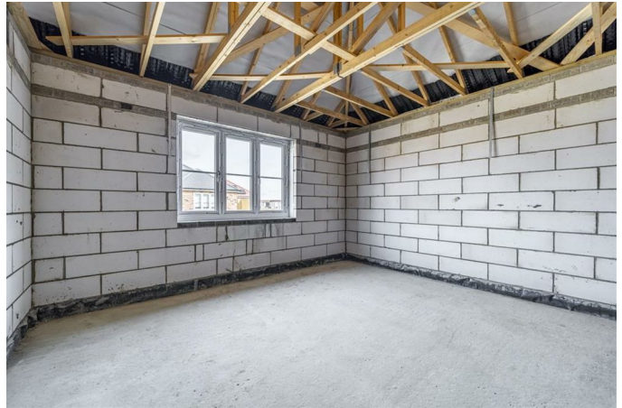
Upvc window to front aspect.
