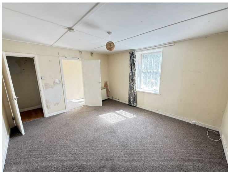
Front window, night storage heater
