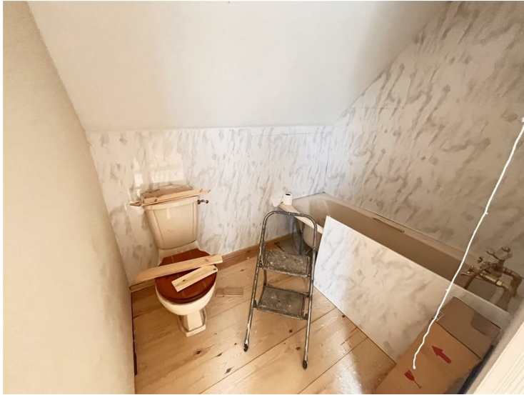
With bath, toilet and wash hand basin
