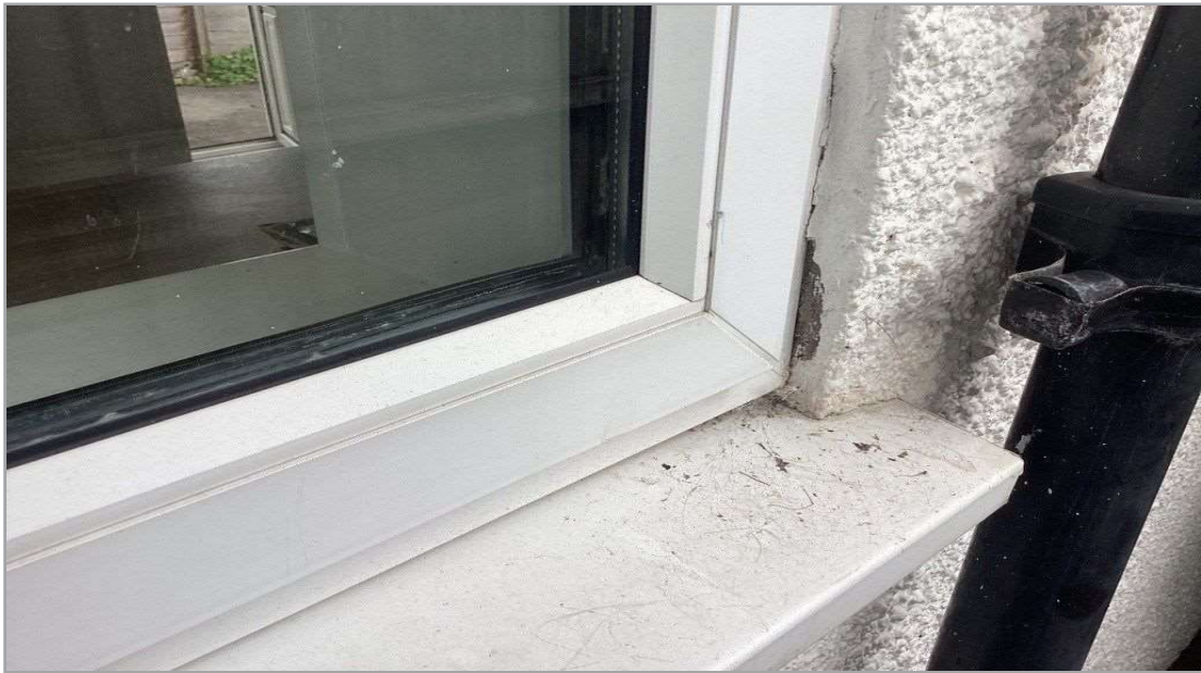
Failing sealant to joints
