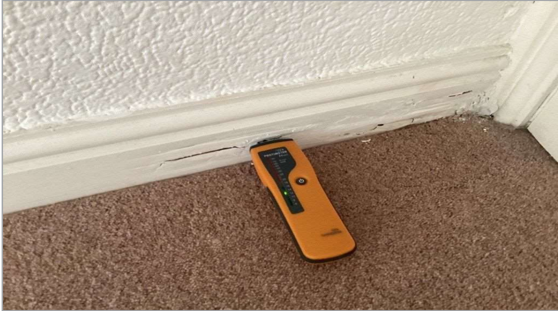
Opposite of bathroom wall and timber rot in skirting behind living room door
