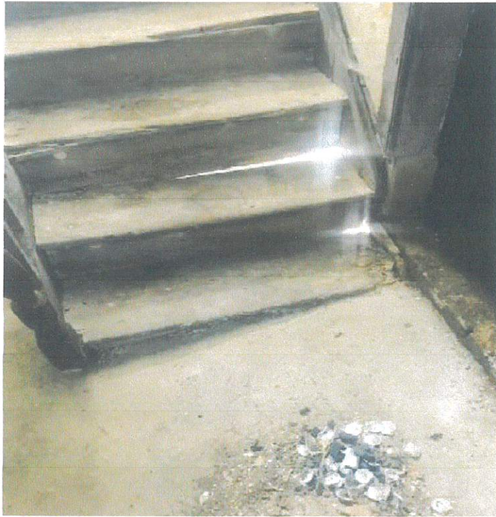
Rot to bottom of timber stair at basement level.
