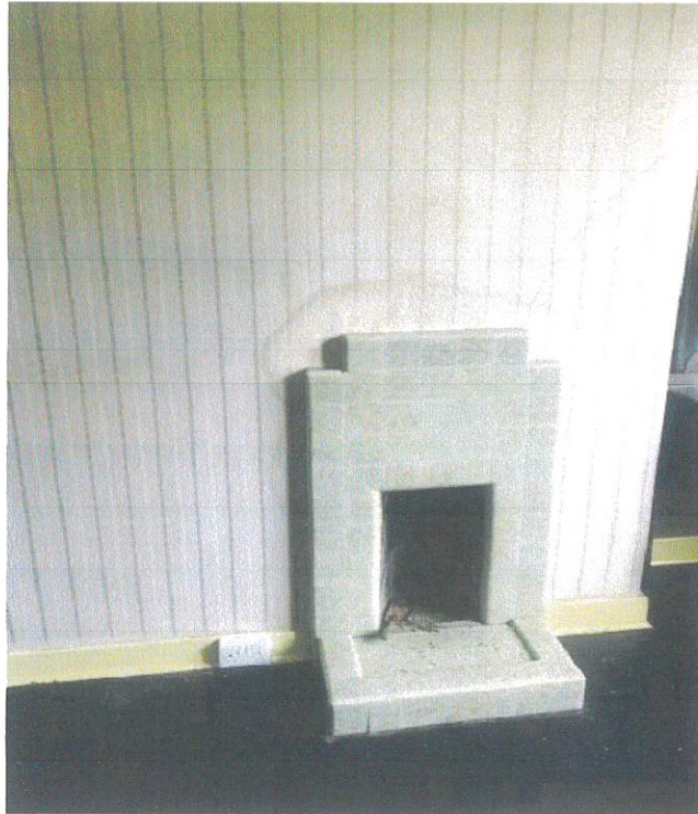
Damp around fireplace.
