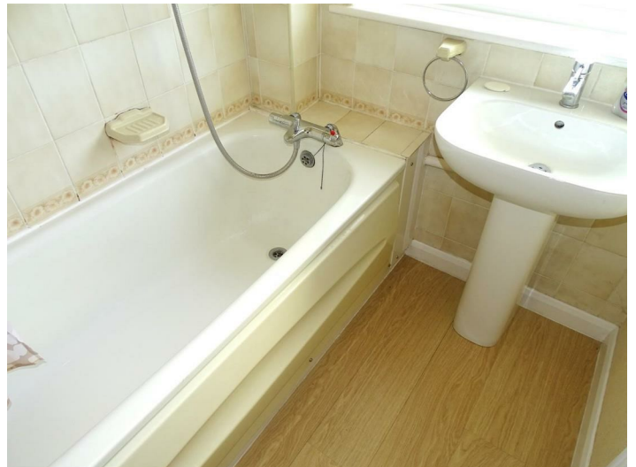
Cast iron bath with shower attachment and tiled wall surround, pedestal wash hand basin, radiator, frosted upvc double glazed window.
