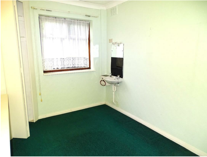
Radiator, aluminium double glazed window, wash hand basin.
