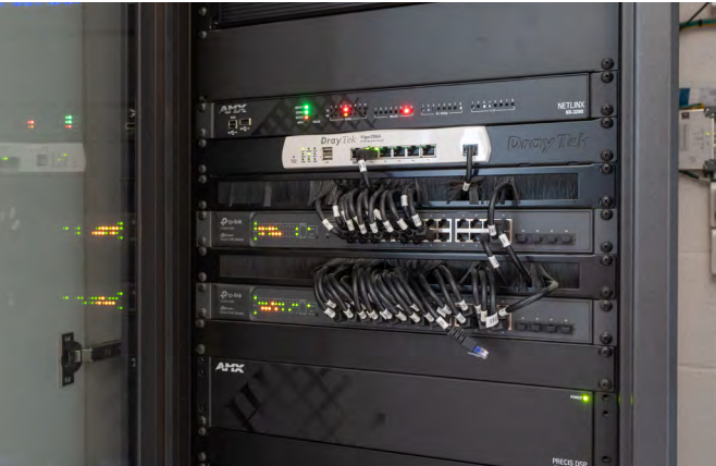
ABOVE: SERVER CUPBOARD
