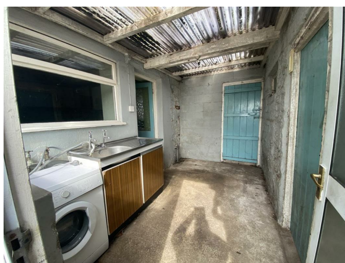
Stainless steel sink and drainer, plumbing for a washing machine, door to outside, door to the workshop.
