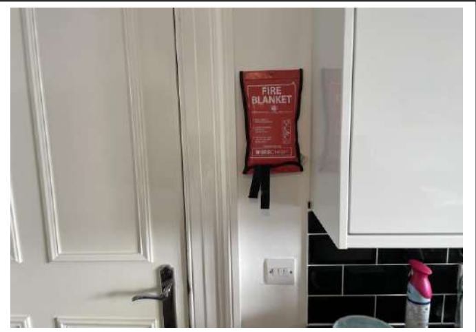
Location – Kitchen Wall
