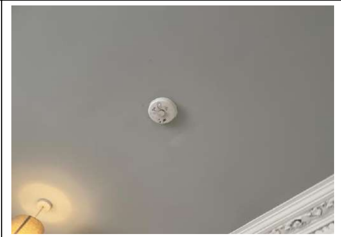
Location – Kitchen Ceiling
