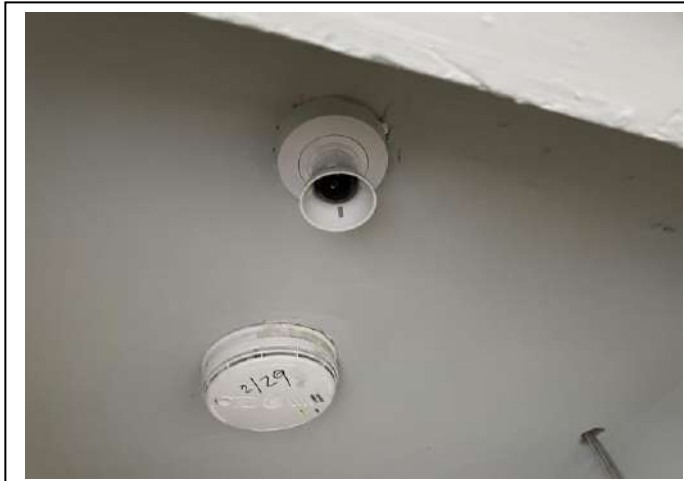
Location – Hallway Cupboard Ceiling
