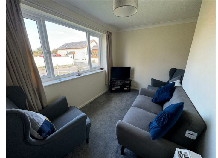
Night storage heater, window to fore.
