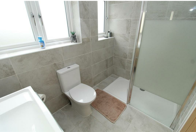
white suite comprising: shower cubicle with electric shower over, wash hand basin in vanity cabinet and low level w.c., traditional radiator, tiled floor and walls, two uPVC double glazed frosted windows to rear aspect
