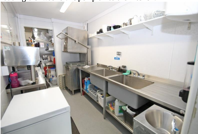
Kitchen Side facing window. Gas cooking range, ovens, fryers, hot plate, griddle and microwave. Stainless steel countertops, shelving units and warming serving unit. Open plan to the dishwashing area. Glass panelled door to the hallway.
