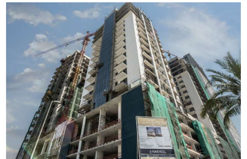
From Left - Right: On - going construction activities of Vita Grande, 7 Park Central and The East Crest as on April 2024.
