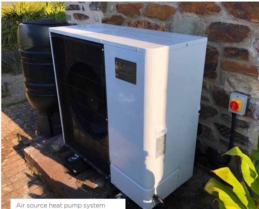
Air source heat pump system
